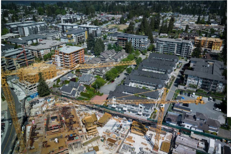
Cranes above a condo development and other housing projects under construction in Coquitlam, B.C. on May 16, 2023.
